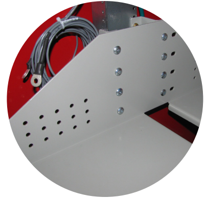
Figure 7: Battery tray screws
