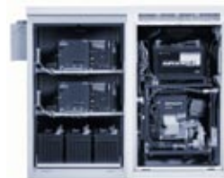
PN-3/CE-3X2 2 Power Supplies 1 Battery String AlphaGen™ Generator
