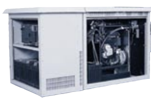
PN-4LSC and PN-4xL 1 Power Supply 36V or 48V Battery Strings AlphaGen 3.5kW or 5kW Generator
