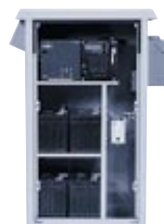
PN-SC-HS Sidecar 1 Power Supply 1 Battery String
