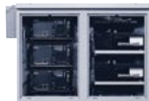
PN-6 3 Power Modules 2 48V Battery strings
