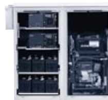
PN-4/CE-9X2 2 Power Supplies 3 Battery String AlphaGen™ Generator
