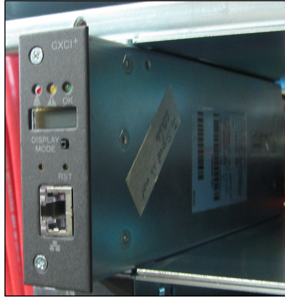
Figure 5—Showing CXCI+ controller module installation
