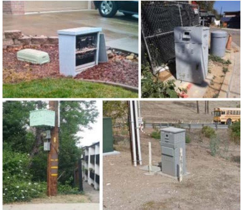
Figure 1: Example cable broadband powering sites. The variability in available space, loading, and local regulations makes a one-size-fits-all solution for extended run time nearly impossible.
