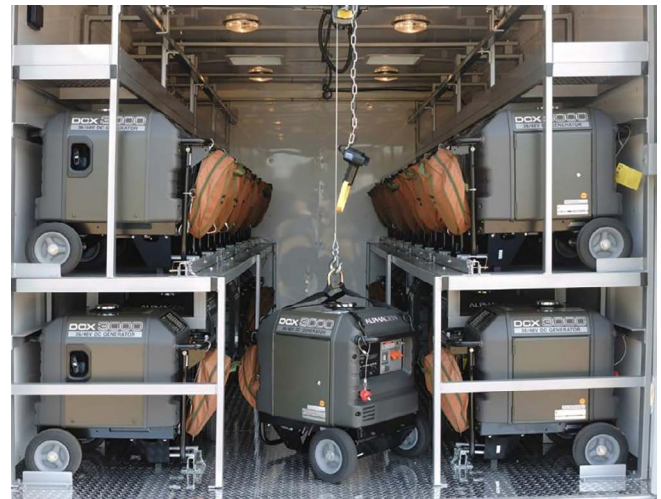
Figure 2: Portable Generators Staged for Rapid Deployment During an Outage
