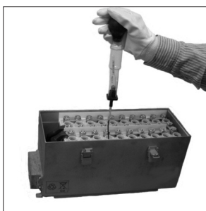
Figure 3: adjusting electrolyte level
